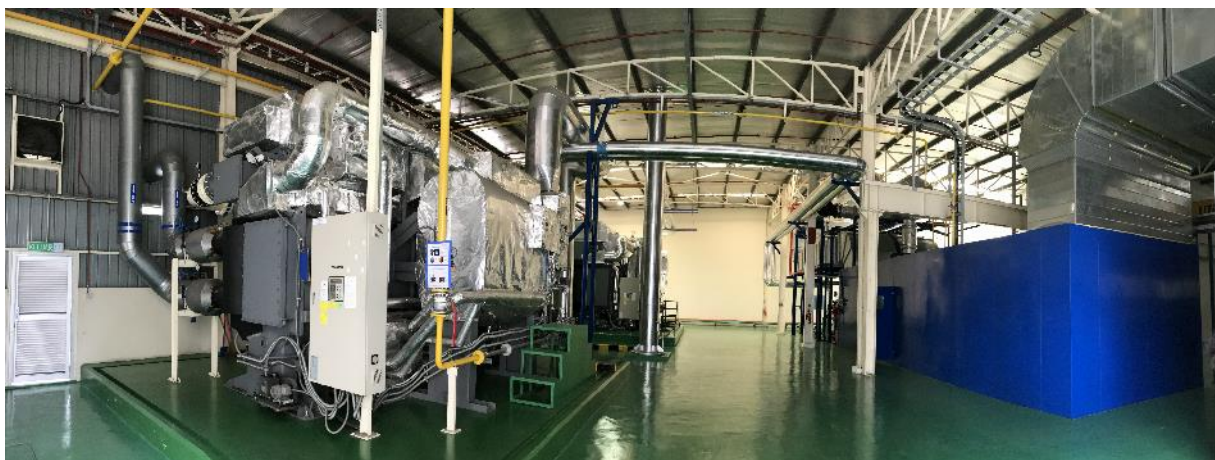
Power generator and air conditioning system at PAPAMY's plant (Right : cogeneration, Left : Genelink)
